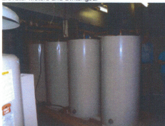
Water Storage Tanks
