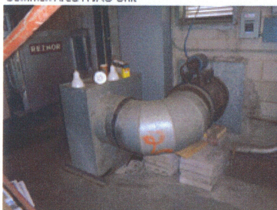
Utility Room Ventilator Fan
