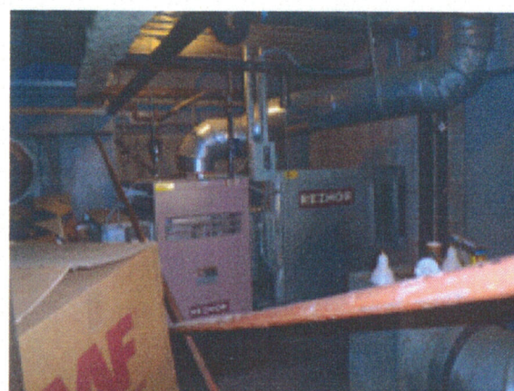
Common Area HVAC Unit
