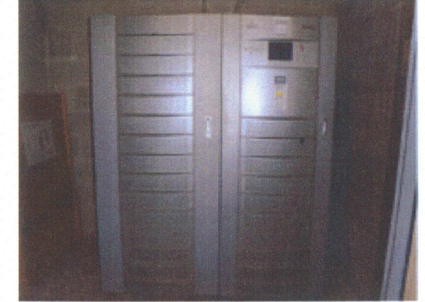
Emergency Power Battery Array
