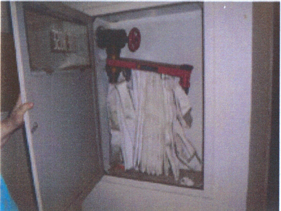
Typical Fire Hose Cabinet
