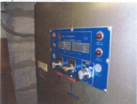
Water Booster Pump Control
