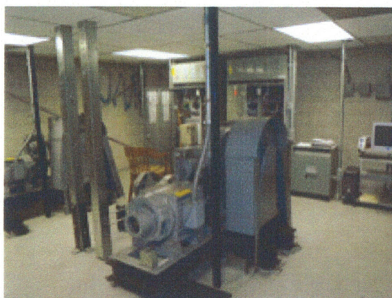
Elevator Motors and Switchgear
