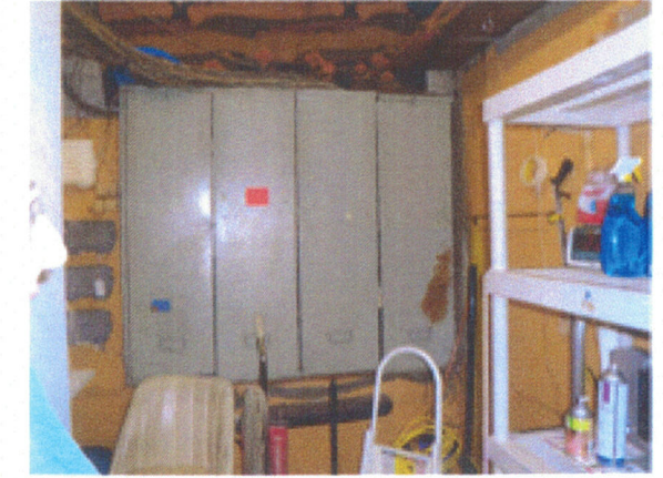
Security System Panel
