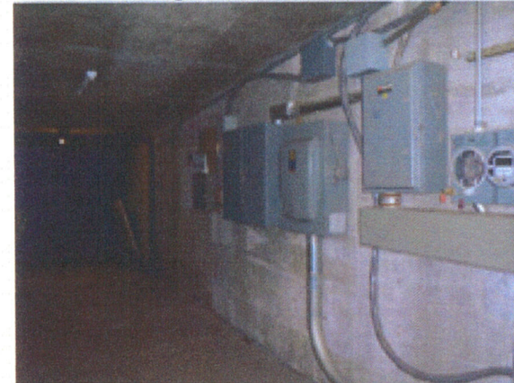
Meter Room Circuit Panels
