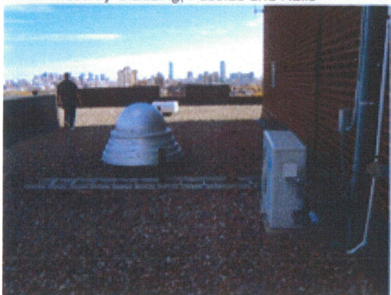
Rooftop Equipment at Mechanical Penthouse
