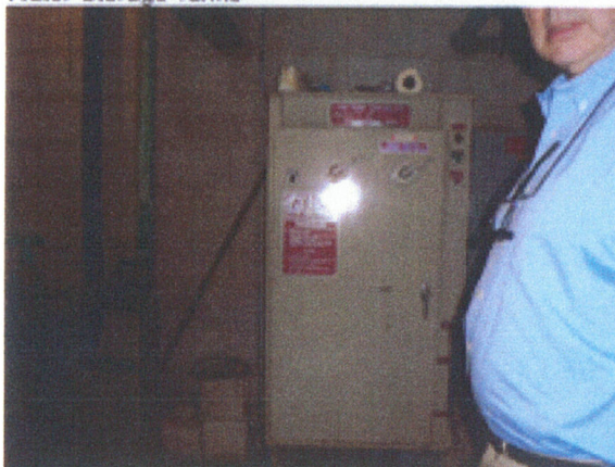
Fire Pump Controller
