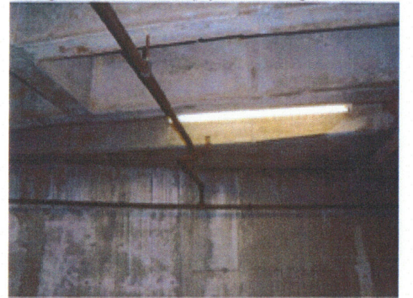
Garage Sprinkler Lines and Lighting
