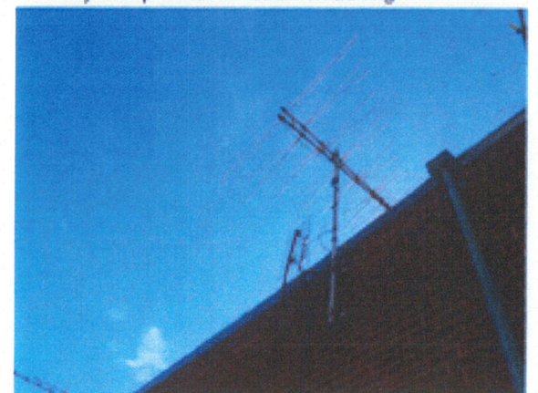
Antennae at Mechanical Penthouse
