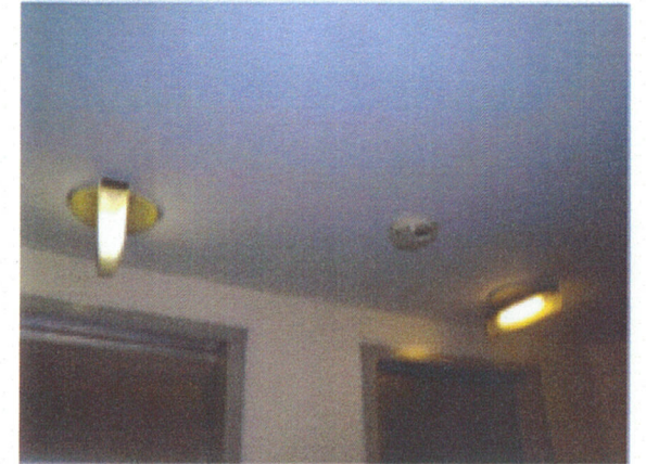
Hallway Ceiling with Smoke Detector
