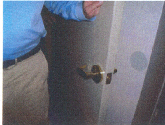
Typical Hallway Hardware
