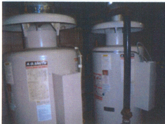
Hot Water Heaters
