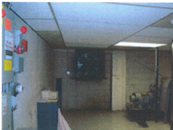
Elevator Control Room
