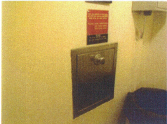
Typical Trash Room Interior
